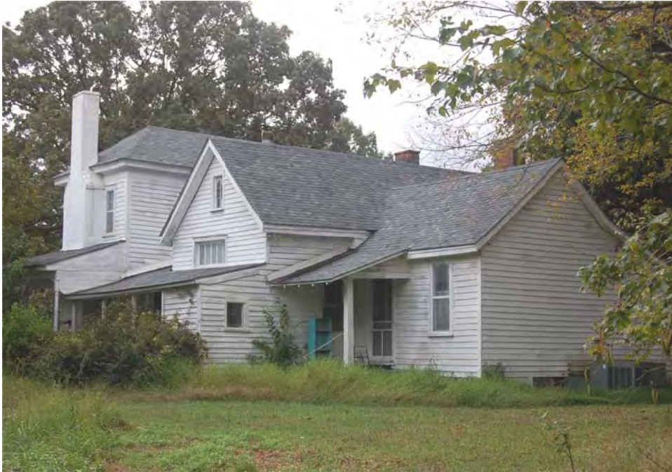
Plate 74. Baucom-Stallings House, Original House, Rear Addition, and Rear Elevation of Main House, Looking South.
