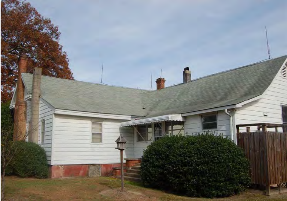
Plate 134. Bell-Pierce Farm, Eastern Tract (WA1252), Bell-Pierce House, Rear (South) Elevation and Rear Ell, Looking North.
