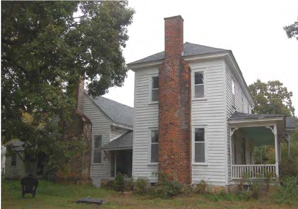
Plate 72. Baucom-Stallings House, Side (West) Elevation and Rear Wing (Original House), Looking East.
