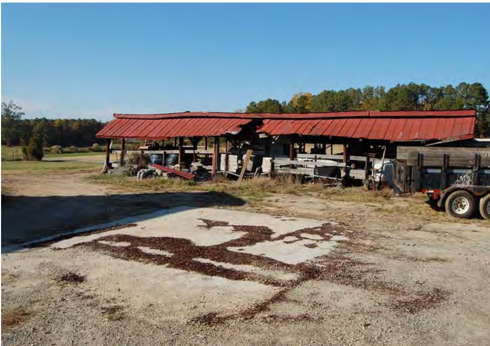
Plate 109. Pierce Farm, Equipment Storage Shed and Concrete Pad (Site of Destroyed Building), Looking North.
